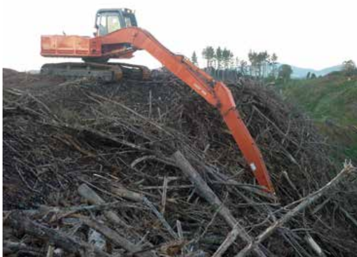
Top, centre, above: A landing failure reduces site productivity, and can trigger environmental effects like highly erosive debris flows. Large boom excavators increase the reach and slash that can be removed. The landing (centre) has had a normal excavator complete the rehab but significant slash remains
