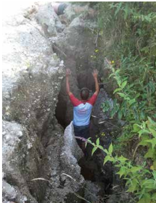
Check ditches for scour. Poor water control maintenance, along with heavy rain and a steep road section, created this bad mix of environmental, health and safety, and infrastructure risk in pumice country
