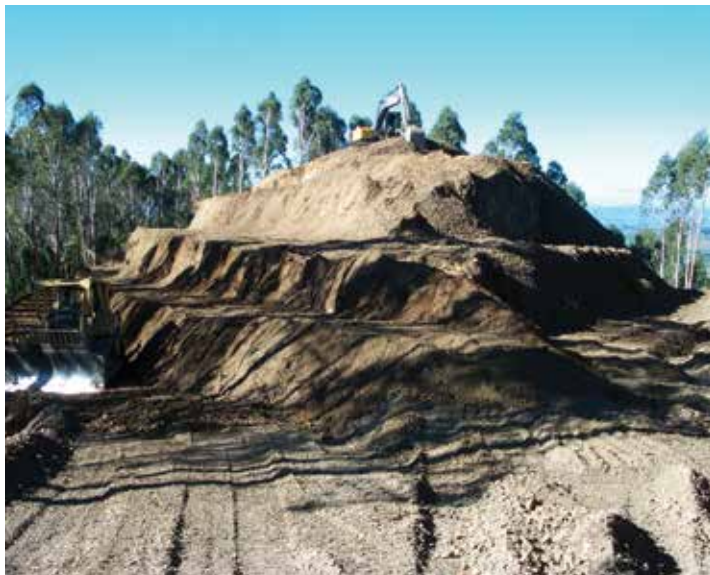
Sometimes large earthworks are required for strategic landings but note the benching established to place the fill. Consider two-staging to reduce earthworks and cost
