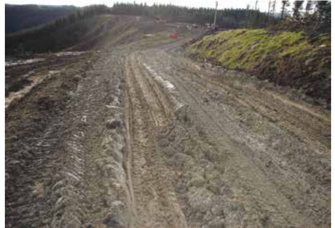
Road rutting creates a safety and maintenance issue
