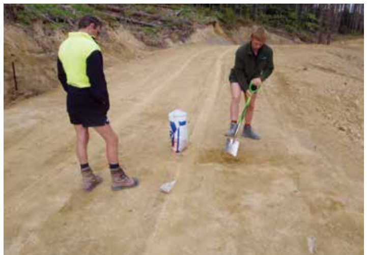
Collecting a soil sample for analysis can provide detailed information about its suitability as an adequate base layer, and can also be used to determine optimal compaction levels
