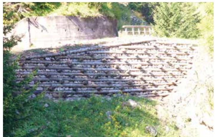
Treated timber crib as retaining wall of forest road fill slope. Never use untreated radiata logs as they are not durable
