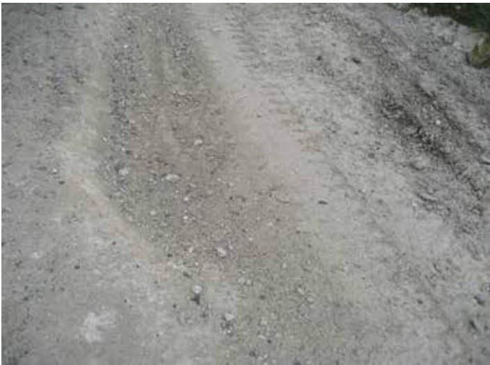
Pavement showing a soft spot
