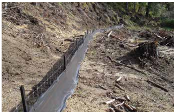
This large silt fence looks well constructed, however the fabric has been installed on the wrong side. It should be on the uphill, so the wire will help support the fabric and stop it from blowing out. The lower edge of the fabric has not been buried because you can see where the sediment has flowed underneath it
