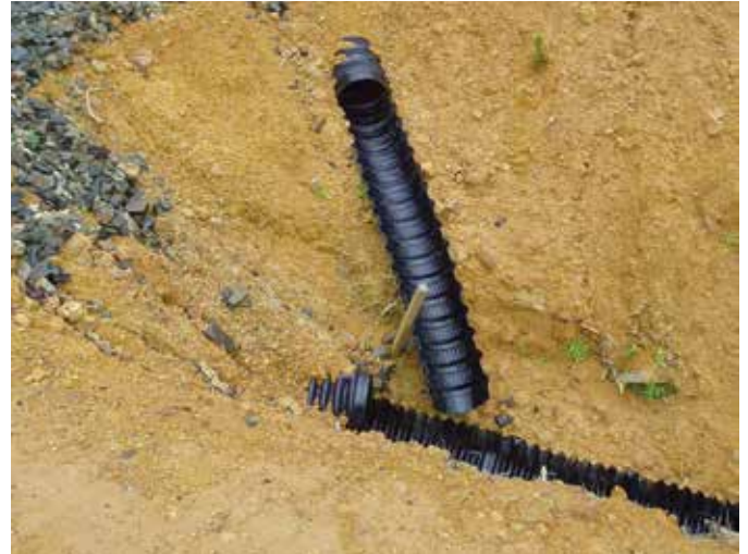
Above: Many components in this image are poor practice. The flume entrance is likely to be bypassed, the flume is poorly pegged, and debris from the slope above is already rolling into the lower flume and partially blocking it. This will create infrastructure and environmental risk.
