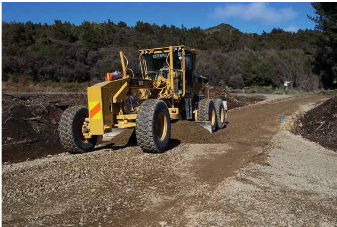
A grader is used to spread the pavement layer over the newly formed road. This layer, when compacted correctly, will provide a good, strong running surface and prevent moisture from infiltrating through to the base course or subgrade layers
