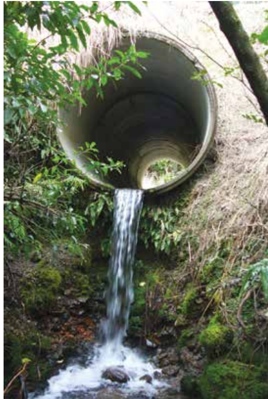
A perched projected culvert eliminates fish passage
