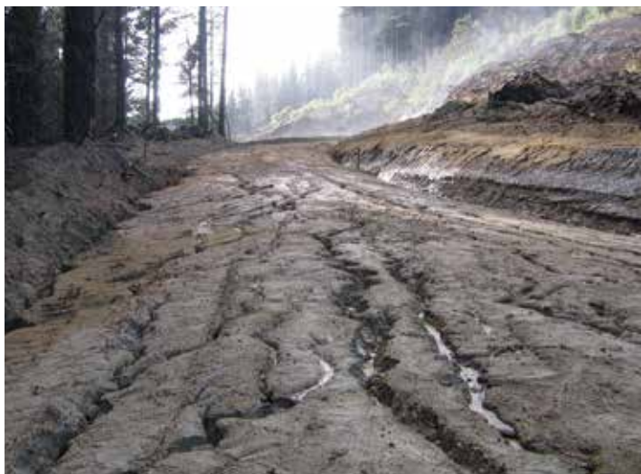
Poor water control during construction can damage a road and cause severe erosion
