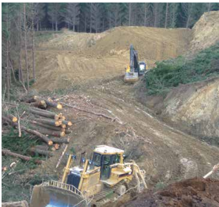
A 37t bulldozer (D8) and a 30t excavator constructing a new road and landing
