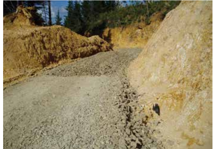
Well-graded material being placed onto the subgrade to form the improvement layer
