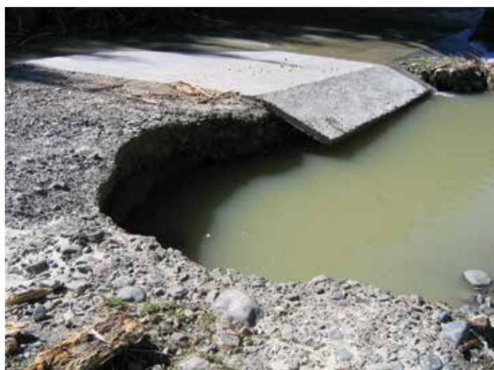
Prompt post-storm maintenance is essential for this structure
