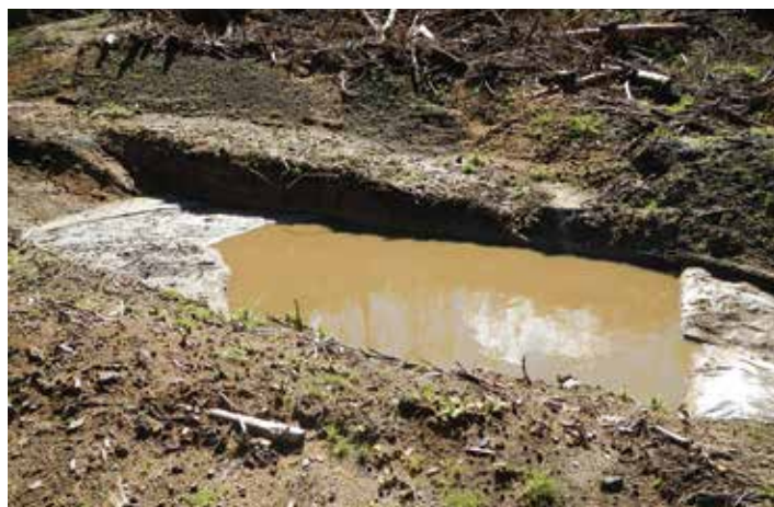
A small sediment pond. It has a low gradient cut-out to the inlet, and is constructed on the hard. It has a broad and flat, cloth-reinforced outlet to slow water
