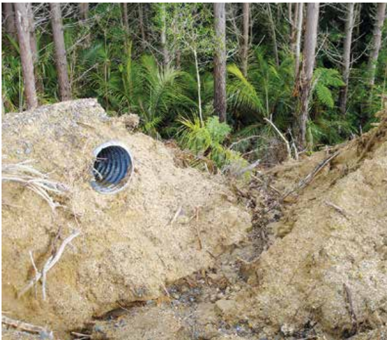
Left: Berm cut-outs can be vulnerable to storm damage because they are compacted fill. Consider armouring, especially when they link to other structures over a fill face, like a culvert sock
