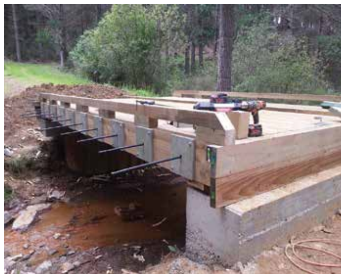
An option to concrete and steel – a New Zealand designed composite post-tensioned treated wood composite bridge
