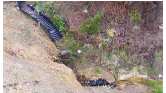
Below: The flume failed because the outlet was not armoured so water undermined and collapsed it
