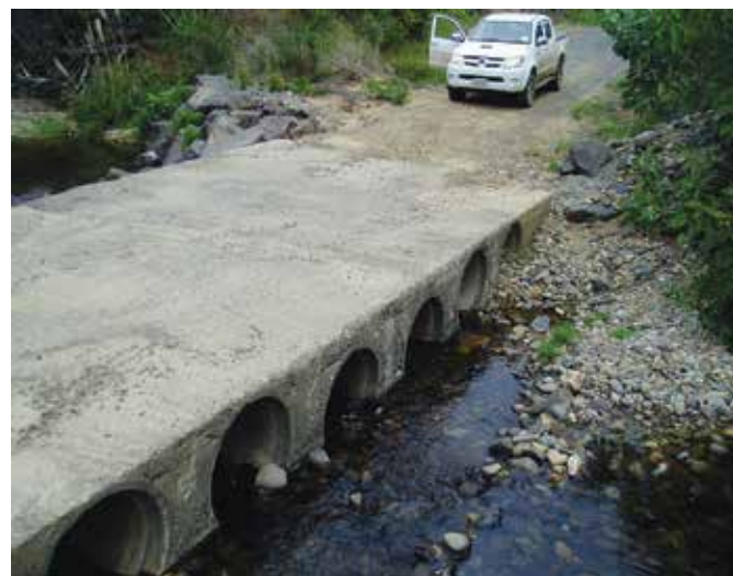
This battery culvert provides for fish passage
