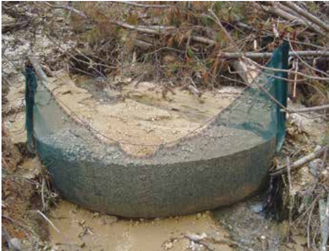
This fence needs maintenance. Sediment is spilling around the sides of the structure
