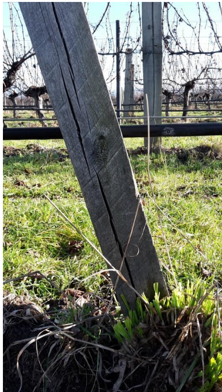
Figure 20: Broken half round CCA pine post in vineyard 2.
