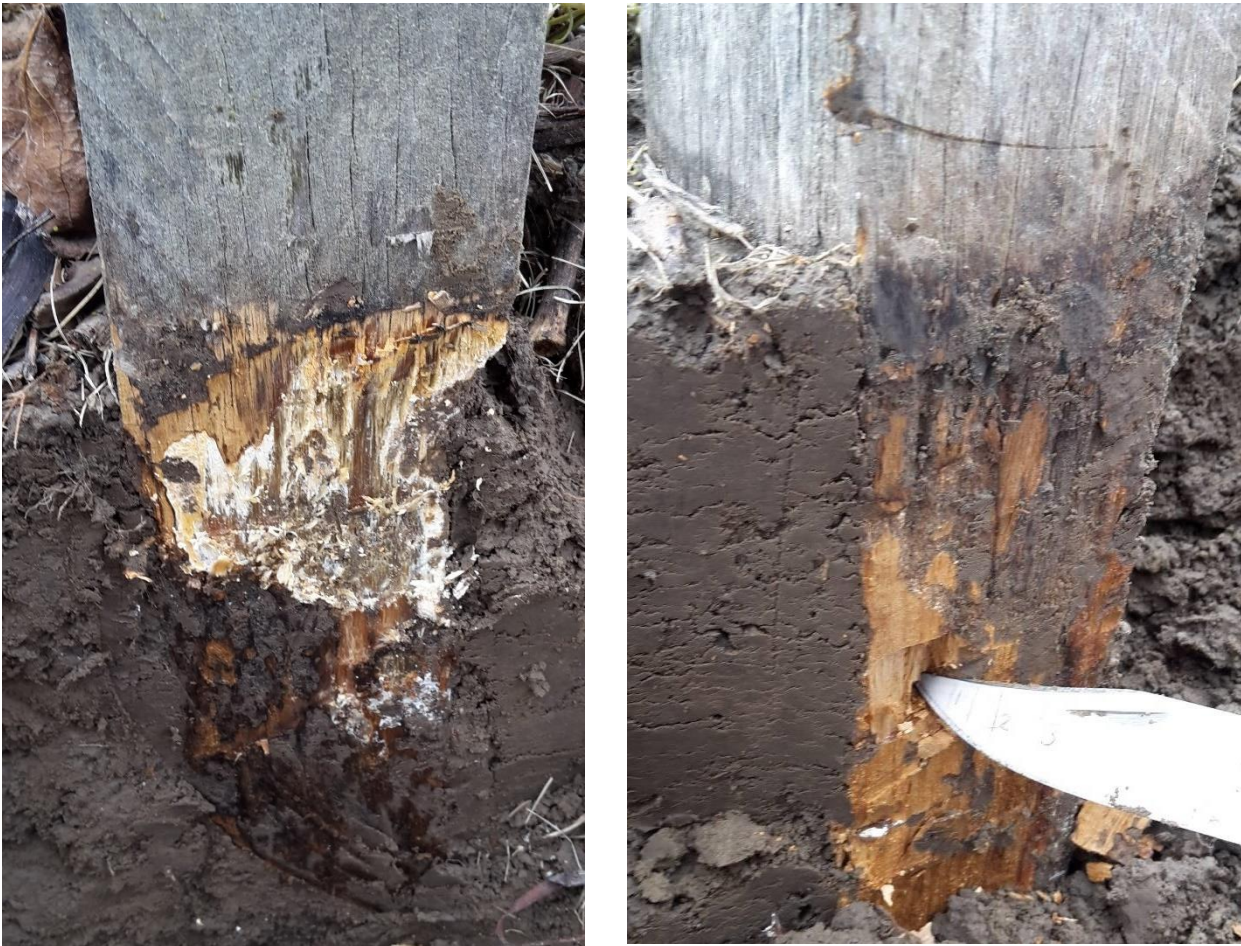
Figure 3: White-rot (left) and brown-rot (right) on E. bosistoana posts after 10 years in service (post 36 and 40)
