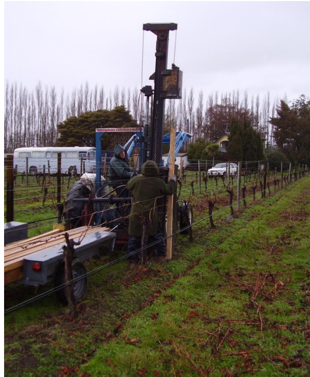
Figure 2: E. globoidea posts being installed in 2007 as replacements for broken CCA pine posts in vineyard 2.
