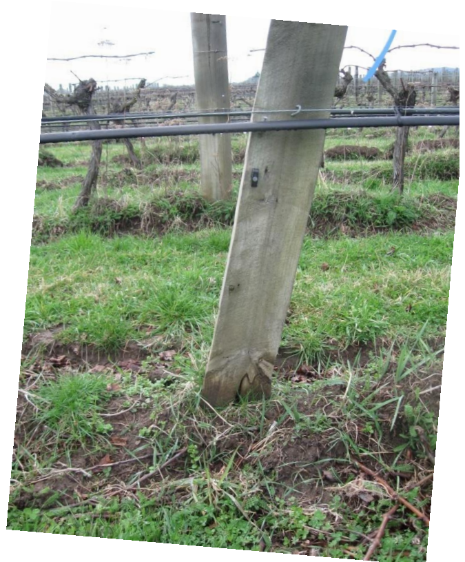
Figure 31: CCA treated pine post cracked across branch whorl at ground level and marked for replacement in vineyard 5.
