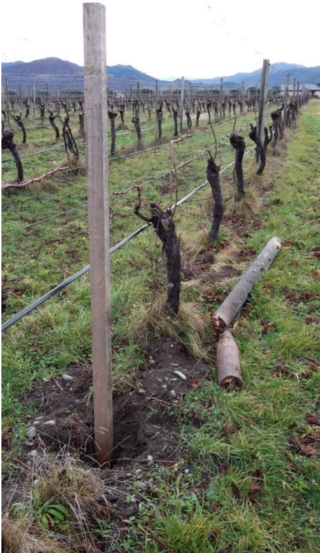
Figure 28: New E. paniculata post being installed to replace broken CCA post in vineyard 4a.
