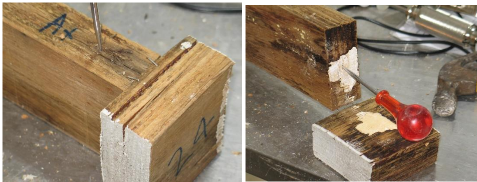
Figure 4: Lightly established decay on the edge and in the joint of untreated Eucalyptus fastigata LVL after one year's exposure (sample 24).
