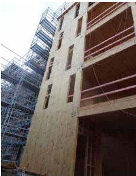
← Figure 6: New medium-rise buildings being constructed using radiata pine CLT, Otago Polytechnic.
